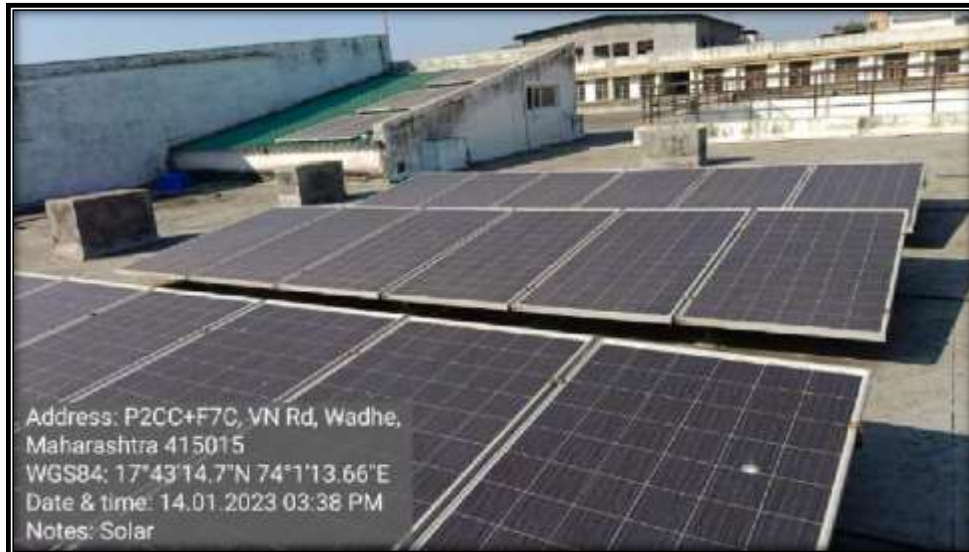
Fig. 7.1.2.1. Solar Energy Panel
